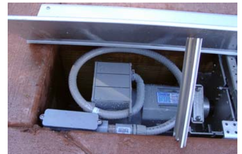
Motor connected to elbow (used as a junction box in this example).
